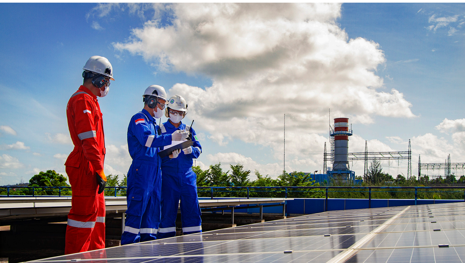
Rooftop Solar Panel, Tanjung Uncang, Batam, Riau Islands Province
