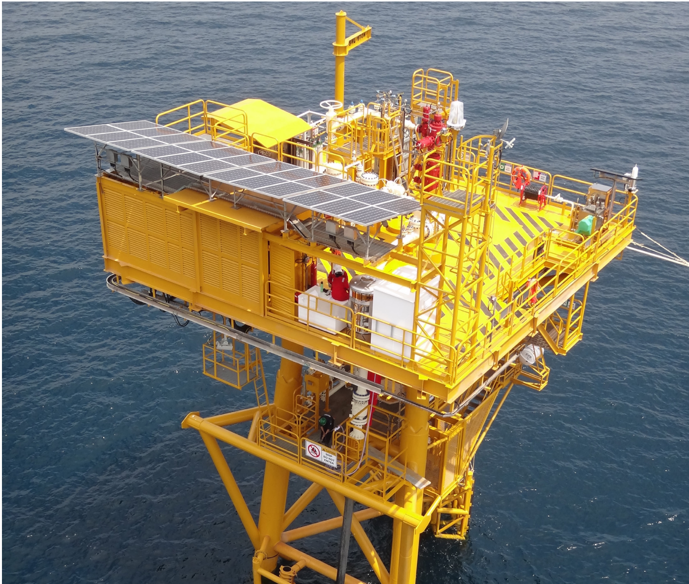
Solar PV at Peluang Wellhead Platform, Madura Offshore, East Java, Indonesia
